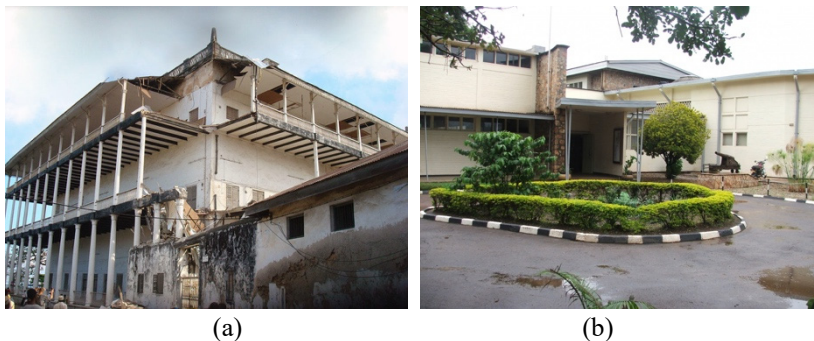
Figure 2: (a) Collapsed corner of the House of Wonders in 2012 [7]; and (b) The Uganda Museum [8].
